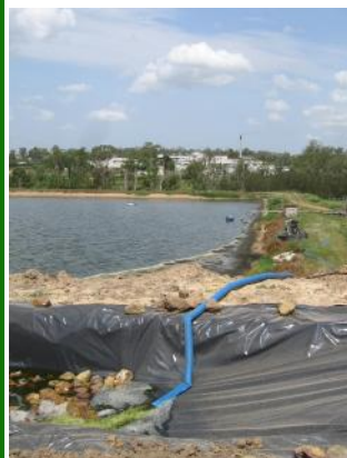
2. Start of a riffle bed nicknamed the "The Trout Stream" to remove Nitrogen, aerate the wastewater, and remove Struvite by crystallisation from the Number 3 Aerobic Lagoon. Build up of sludge around the margins indicates that the ponds are overloaded which would eventually create anaerobic conditions in the aerobic pond.
