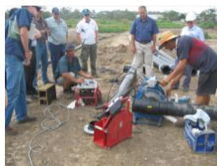
9. Pipe welding techniques being demonstrated. A key point was that each weld takes about one hour to complete; other issues of weather, dust, cleanliness etc were also discussed.
