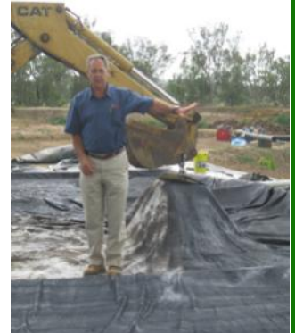
11. One method of achieving a 'lift' of the cover to avoid pooling of water. This method has now been discarded. Note that the cover material can be damaged but is readily and easily repaired in-situ compared to HDPE.
