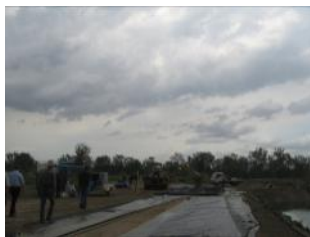
8. Demonstration of the Liquid Rubber pond cover that is being trialled. Unfortunately the rain beat us before an application demonstration could be done.
